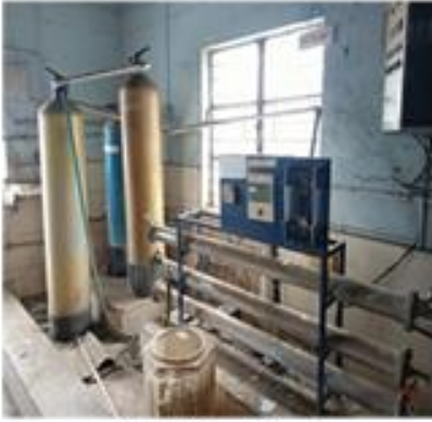
RO Water Plant
