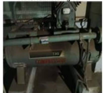
Air Compressor Unit
