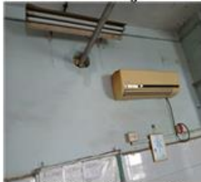
Split Air Conditioning Unit
